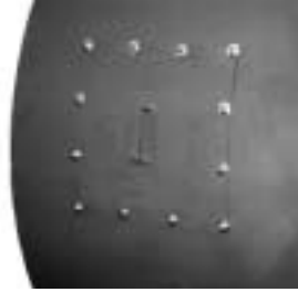
Bolted Access Door
